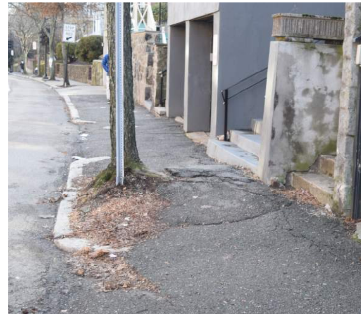
Tree roots heaving sidewalk
